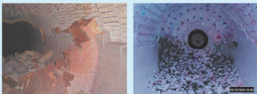
Fig 1: Typical extreme refractory failures
