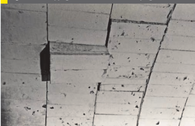
Fig 5: Brick slippage due to insufficient keying action
